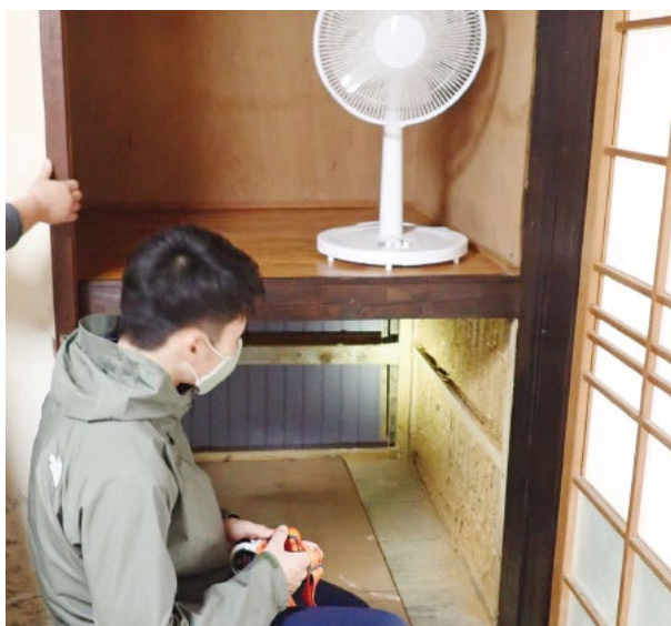
▲Affected house with closet opening leading to exterior wall.
